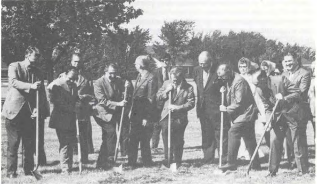
It was June 17, 1971, and the first shovels of earth were turned for new dormitory facilities at the Hastings Campus. Those turning the first shovels are from left to right: Verne Moseman, Board of Governors member from Grand Island; John McGinley, First National Bank, Hastings; Hastings Mayor William Geltman; Shorty James, Carmickel Construction Co.; Ed Minnick, Campus Dean of Students; and College President, Dr. Chester H. Gausman.
