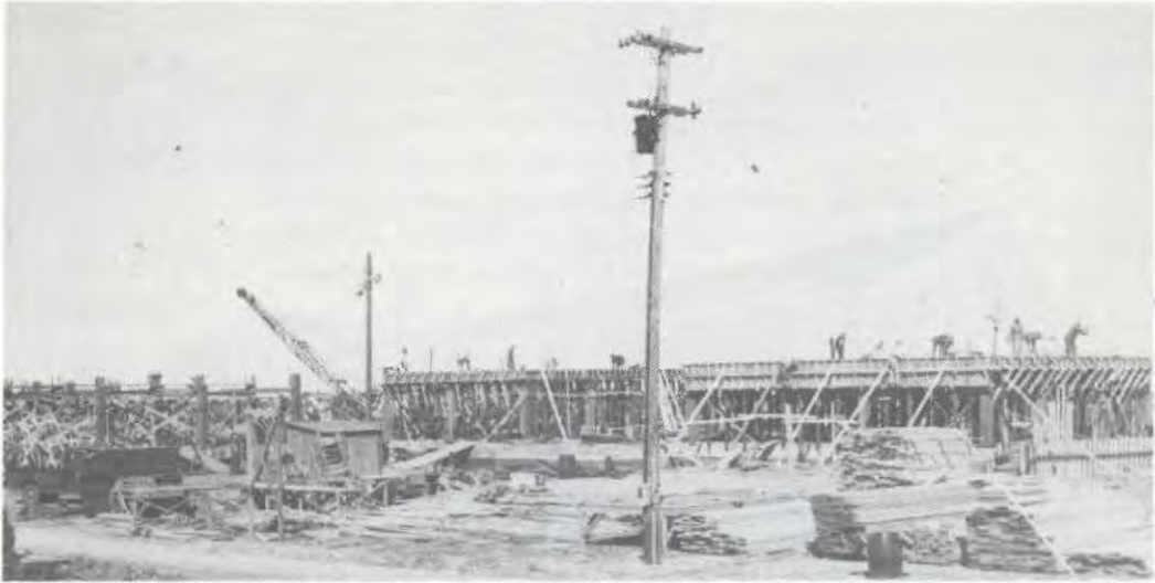
Under construction in 1943 is building #5. This building would serve the Navy as a barracks, and later the college, first as a dormitory and classroom building and then as an instructional facility.
