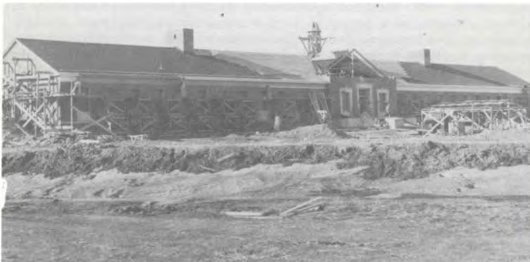
The Naval Ammunition Depot administration building under construction in 1943. This building would serve the college as a dormitory and classroom building.
