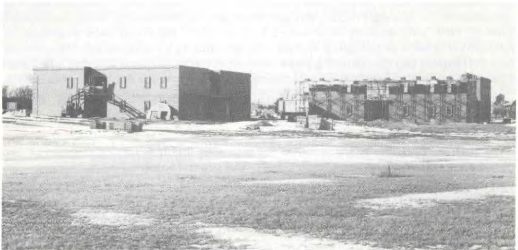
Work continued throughout the winter on two dormitory buildings financed through the issuance of revenue bonds.
