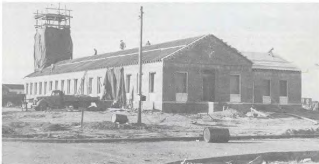
The Navy laundry building under construction in 1943. When the building was received by the college, it was renamed the Phelps Building.
